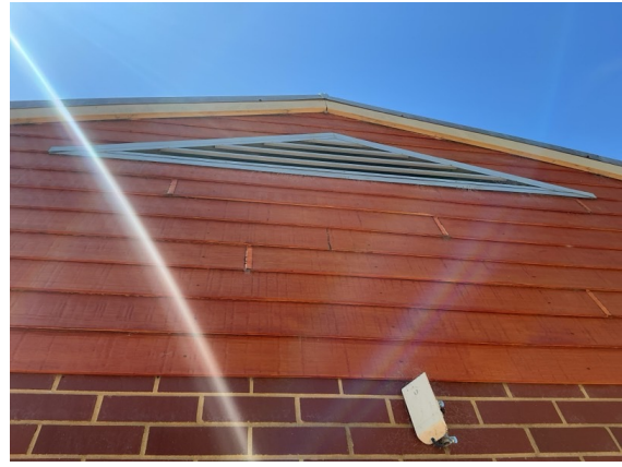
Deterioration noted to the north and south elevation gable weatherboards. Recommend maintenance/ repairs.
