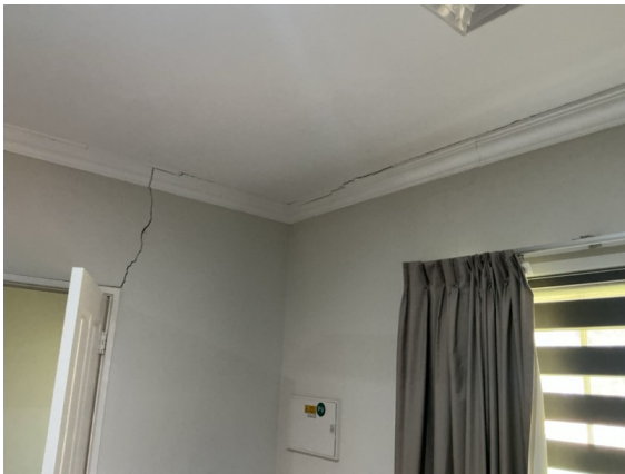
Bedroom 1/ entry wall - Vertical cracking
