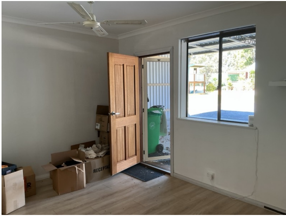
Entry - Recommend council record search for all shed additions and living areas.
