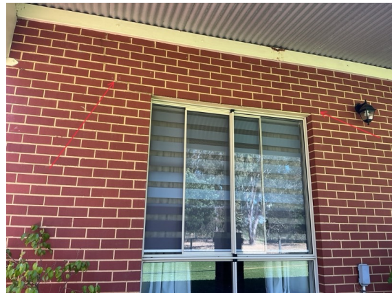
Southeast corner - Evidence of step and vertical cracking which has been previous repaired. Recommend review by qualified tradesman and repairs as required.
