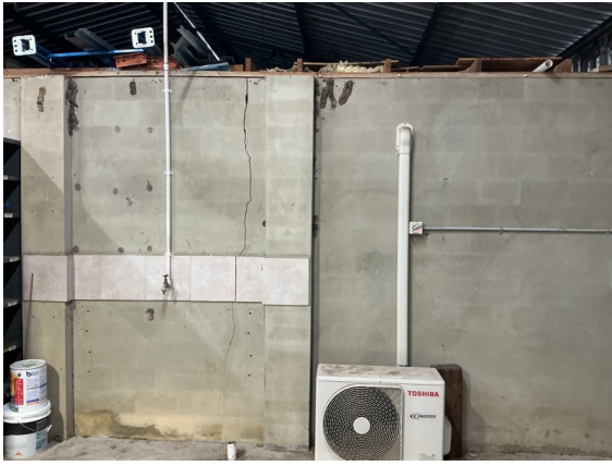
Southeast elevation - Vertical cracking observed to various areas of the shed living areas. Recommend repairs or seek further advice from a Structural Engineer.
