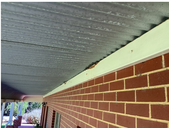
Surface rust noted to the exterior roof sheets and steel framed roof members at the crack line between the house and verandah on the east elevations. Recommend maintenance/repairs.
