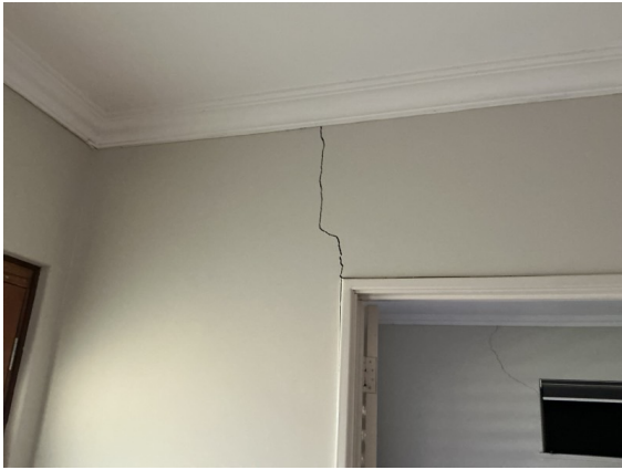
Entry - Evidence of cracking noted to various interior areas. Recommend repairs or seek further advice from a Structural Engineer.
