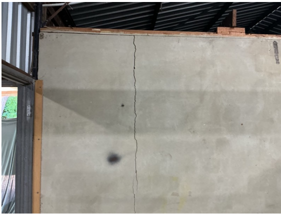
Southwest elevation - Vertical cracking observed to the shed living area.
