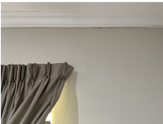
Bedroom 1 - Cracking adjacent to east elevation exterior noted in defect 2.
