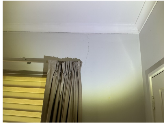
Bedroom 3 - Cracking adjacent to Northeast elevation exterior cracking noted in defect 2.
