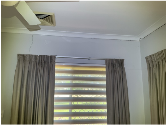
Bedroom 3 - Cracking adjacent to Northeast elevation exterior cracking noted in defect 2.
