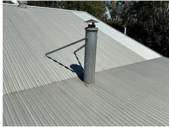
There is no dektite installed to the alfresco fire place flume. Recommend installing a fire rated dektite and silicone.
