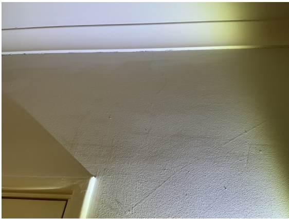
Typical appearance cracking noted to rendered walls at some isolated areas throughout the home. Recommend maintenance/repairs.
