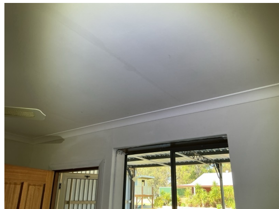
Typical appearance cracking noted to the ceiling junctions at some isolated areas throughout the shed. Recommend maintenance/repairs.
