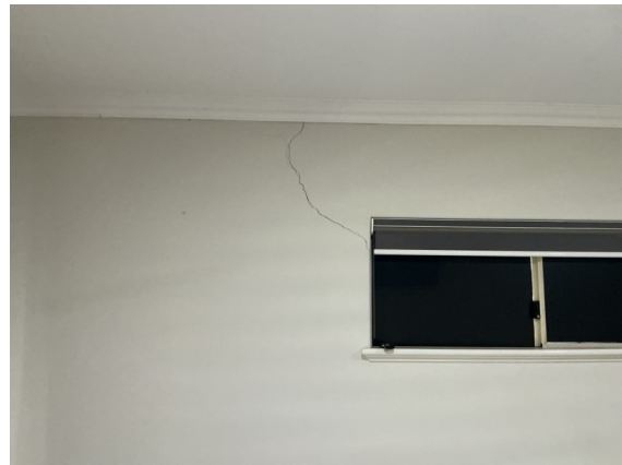
Bedroom 1 - Cracking adjacent to south elevation exterior noted in defect 2.
