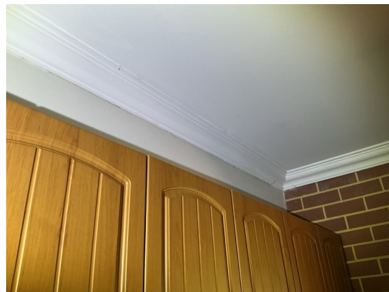
Typical appearance cracking noted to the cornice at some isolated areas throughout the home. Recommend maintenance/repairs.
