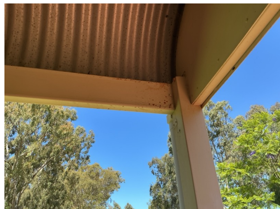
Surface rust noted to various steel posts and beams on the east and west elevations. Recommend maintenance/ repairs.
