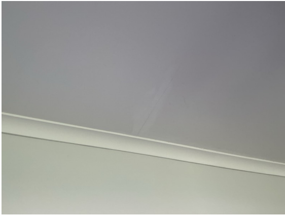
Typical appearance cracking noted to the ceiling junctions at some isolated areas throughout the home. Recommend maintenance/repairs.
