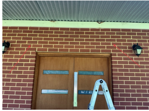
Entry - Evidence of vertical and step cracking noted above the entry door.
