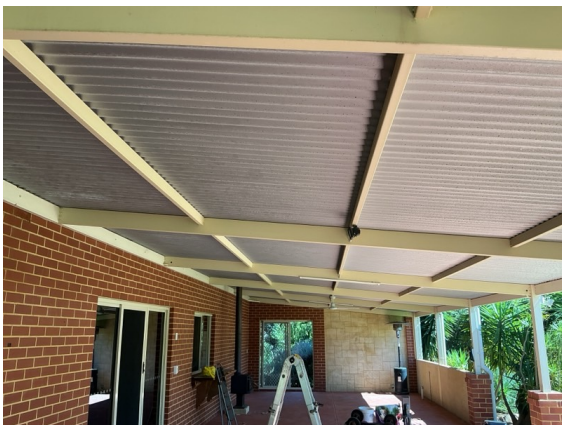
Patio connections were performing on day of inspection.
