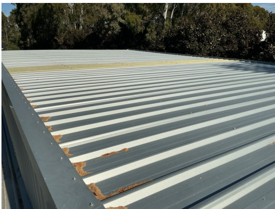
Minor deterioration noted to the fibreglass skylight sheets. Recommend maintenance/repairs.
