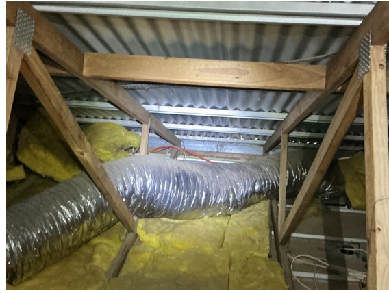
Premier tie down straps observed.
