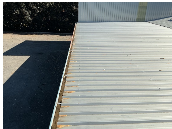
Debris in the gutters on various elevations. Recommend keeping the gutters and down pipes clear to allow adequate flow to the storm water system.
