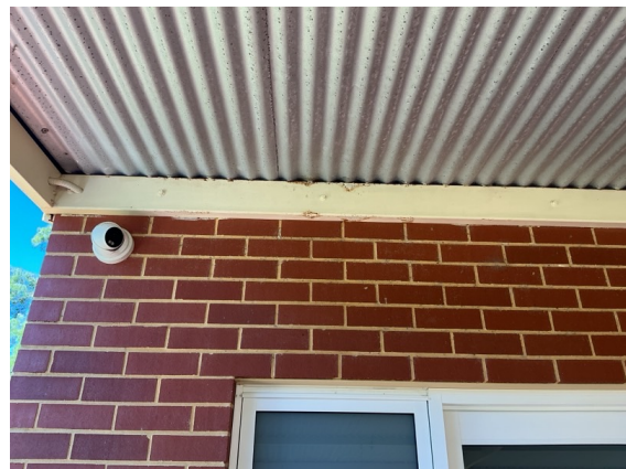
Surface rust noted to the exterior roof sheets and steel framed roof members at the crack line between the house and alfresco on the west elevation. Recommend maintenance/repairs.
