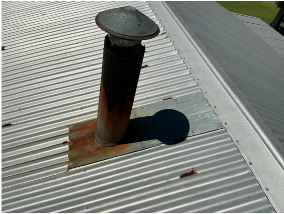
Deterioration to the roof flume on the west elevation. Recommend replacement.
